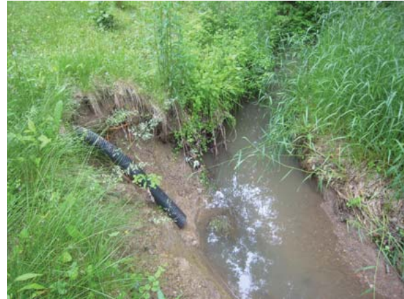
Stormwater drainage, such as this residential drain pipe, can cause stream bank erosion.
