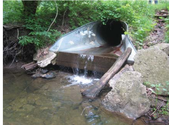
Erosion around a stormwater outfall, Rock River Ravines.
