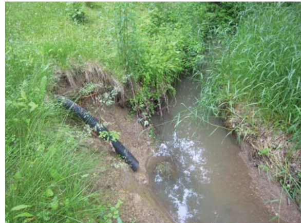
Stormwater drainage, such as this residential drain pipe, can cause stream bank erosion.
