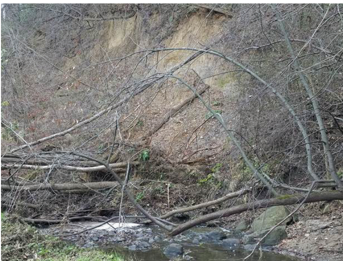
This is the stream bank that will be stabilized. As you can see from the image, there is a need to clear fallen trees and thin the canopy to encourage ground vegetation growth and reduce erosional concerns along Blackhawk Creek.
