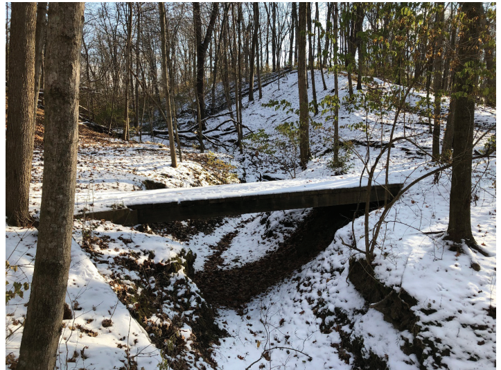
This is one of two bridges that will be replaced on the Sac Fox Trail at Loud Thunder Nature Preserve.
