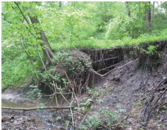
High flows can cause stream bank erosion and loss of property.
