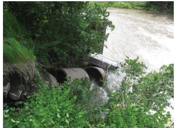
DW 13: stream bank erosion can cause the failure of stormwater infrastructure, requiring expensive repairs.
