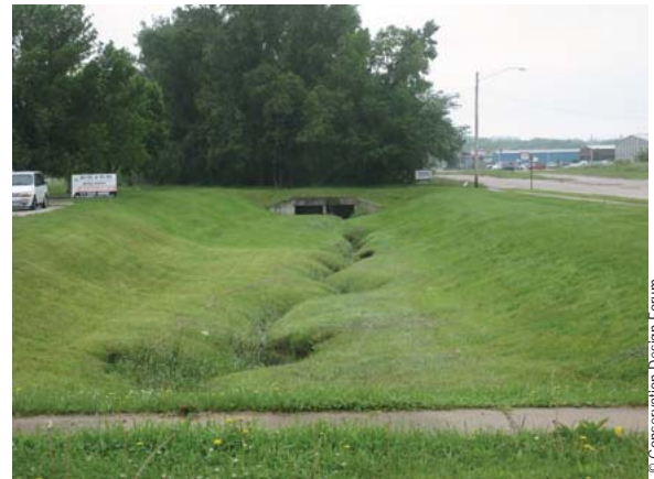
RR7.5: evidence of early stream downcutting within this turf grass stream corridor.
