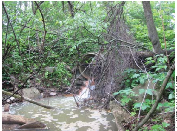
RR6.4: a stormwater outfall causing erosion.
