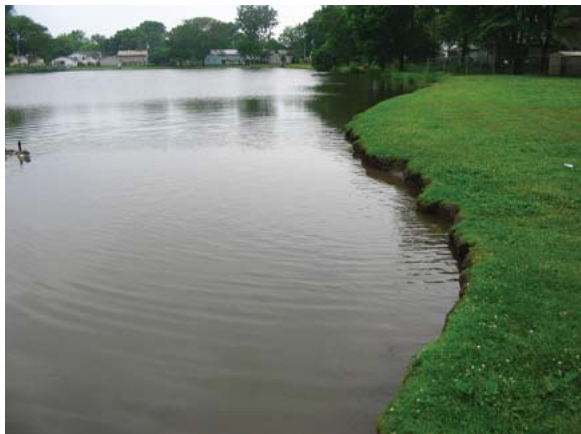
RR8.1: eroding banks of this detention basin contribute to water pollution.
