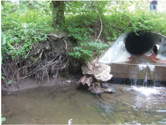
RR5.10: erosion around a stormsewer outfall.
