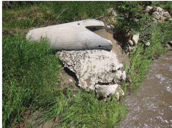
RR2.3: water flow from stormwater outfalls commonly causes erosion.
