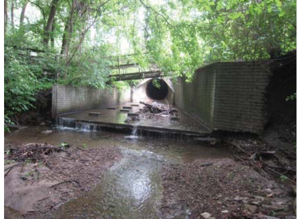
RR8.2: massive erosion and stream destruction at this culvert.
