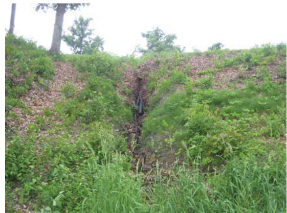
RR10.7: these plastic drain pipes are causing erosion.
