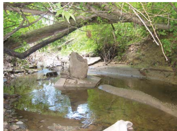
RR2.13: erosion at stormwater outfalls can cause stormwater infrastructure to fail and become dislodged, requiring expensive repairs.
