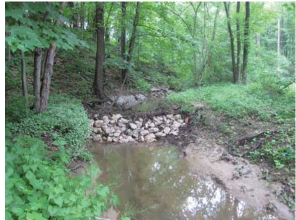
RR7.7: an attempt to halt stream channel and bank erosion.
