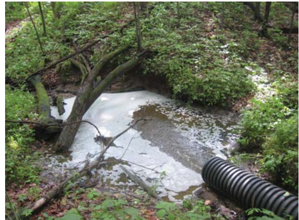
RR10.6: this stormwater discharge is eroding away a pool below the outfall.
