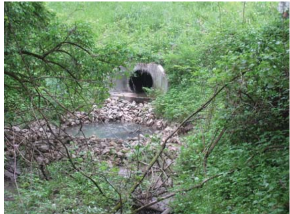
RR8.7: an attempt to reduce the erosive energy of this stormwater outfall.
