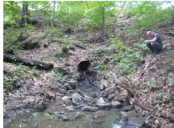
RR2.9: stormwater culverts under roads are common points of erosion.
