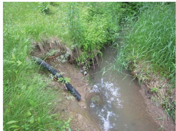
RR7.7: a residential drain pipe causing erosion.
