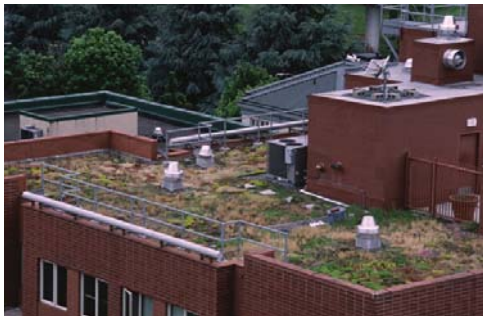
Green Roof (Portland, OR)
