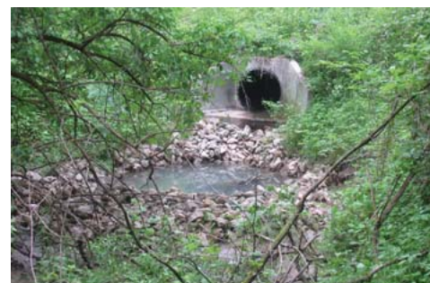
an attempt to reduce the erosive energy of this stormwater outfall
